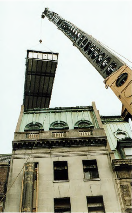
The pool being lowered onto the roof (above) and (right) ready for laps. The marble fountain (outside, on the terrace) and the statue of Mars, both English, are in the classical manner.
